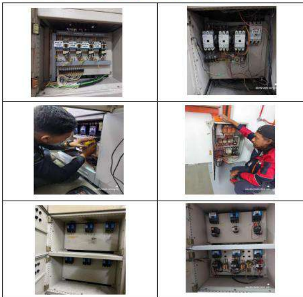
3. Dismantle and dispose electrical panel, component and others related at Jotun Paints Malaysia.
